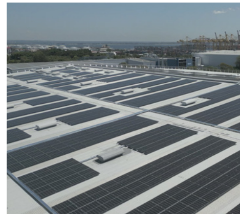
The solar installation at the Matraville factory.
